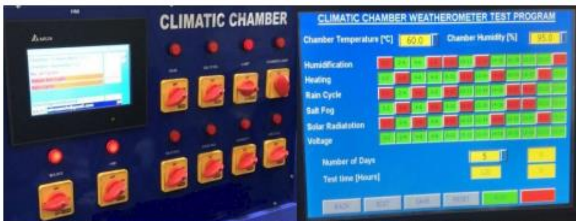
Fig.7 Control arrangement and Input panel (developed HMI system for Multistress)
